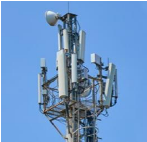
Antenna Base Station(RRU)
